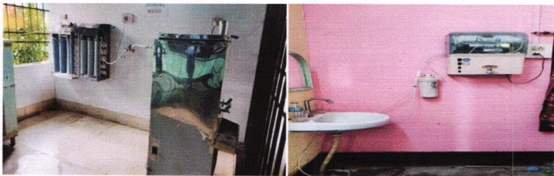
Figure: Drinking water facility
