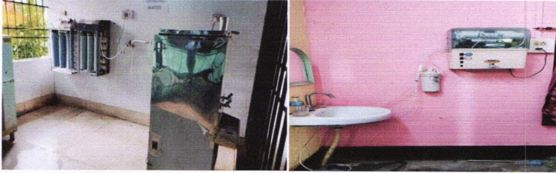
Figure: Drinking water facility
