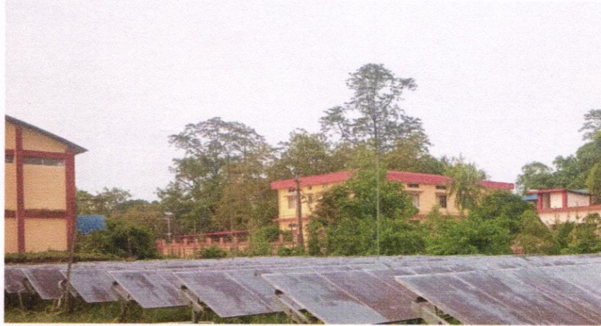
Figure: Alternative power generator 50 KW
